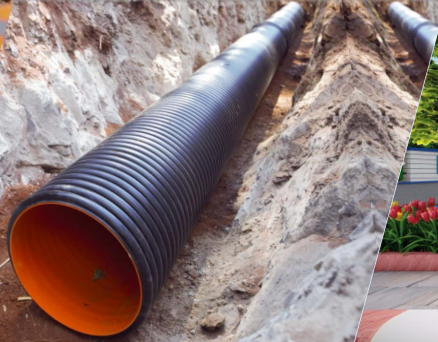
Underground Sewer Pipe Line
