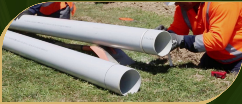
Water Pipe Line
